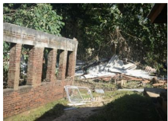
Postmortem Room with Destroyed Roof which was erected before 2 weeks
