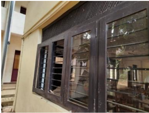
Damaged Windows of the Canteen Building
