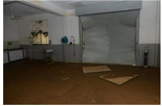
Entrance Door, OPD, VTH-FA
